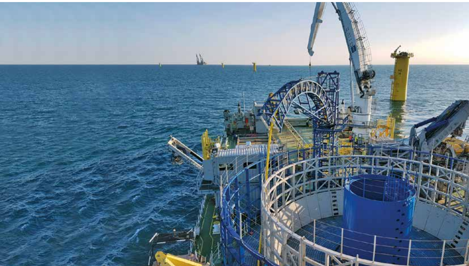
Offshore installation of TKF 33 kV subsea inter-array cable for the Hohe See wind farm in the German North Sea, approximately 95 kilometres North of Borkum. The offshore wind farm installation project in 2018 covers 71 turbines in an area of around 40 square kilometres with water depths up to 40 m. The wind park has a capacity of 497 MW and a total of 52 km subsea cables was installed.
